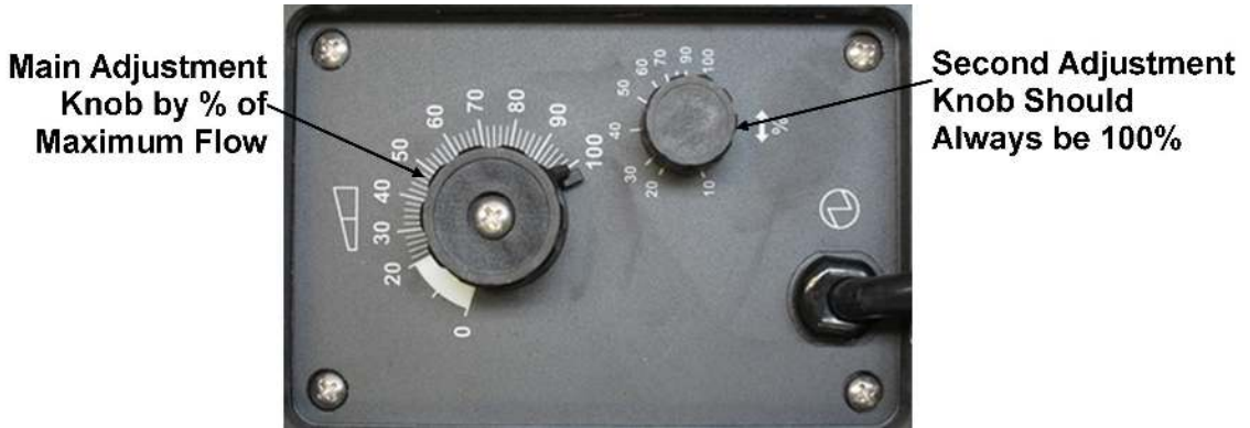
Fig. 4 – 5: Rinse Injector Pump Controls
