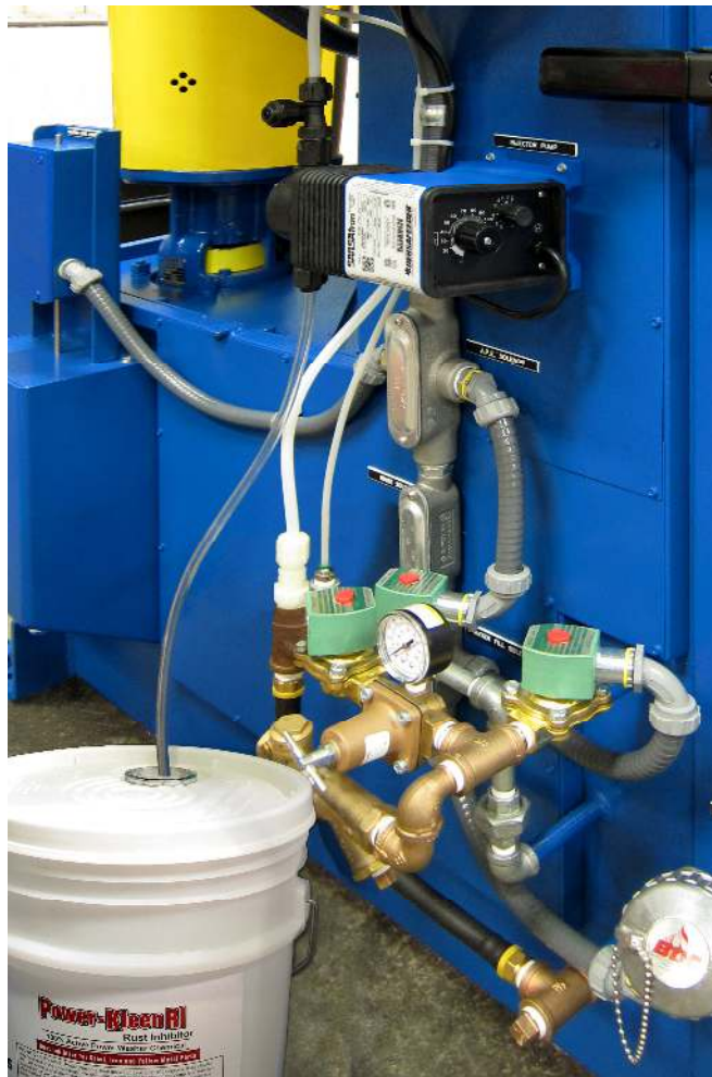
Rinse Chemical Injector System
