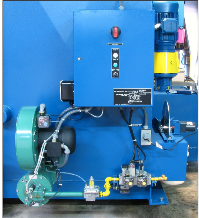
Retrofit Burner installed on MART Washer
